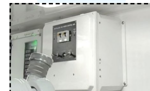
Sample Pump Control
